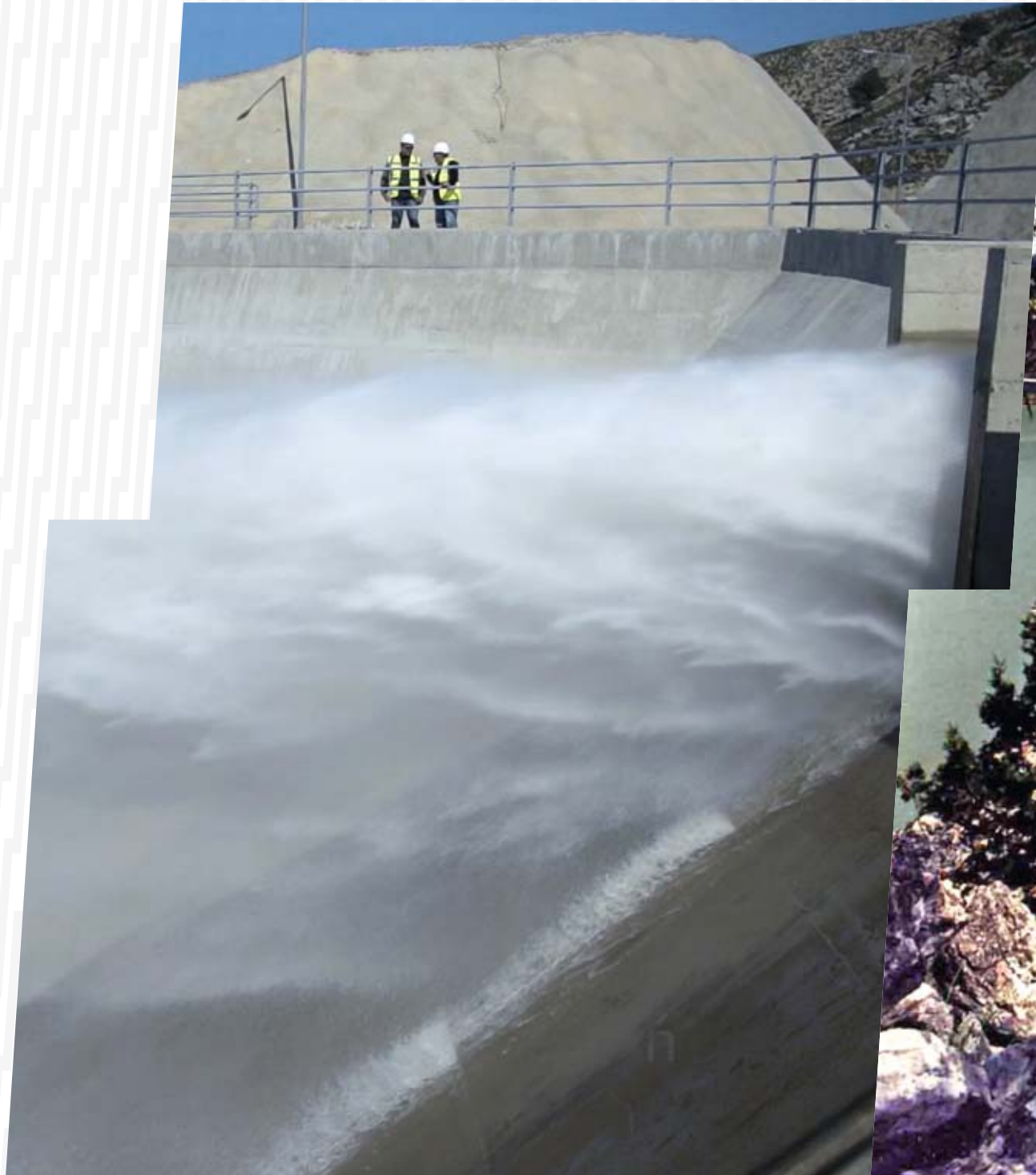
Hybrid energy project of Ikaria, Naera
