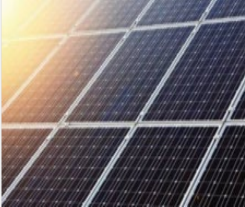
Project: Ptolemaida (PV) Location: Ptolemais - Region: West. Macedonia Capacity: 171MW Status: Under Construction
