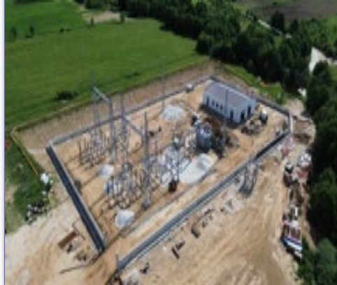
Project: Doukas (WP) Location: Ptolemais - Region: West. Macedonia Capacity: 26MW Status: Under Construction
