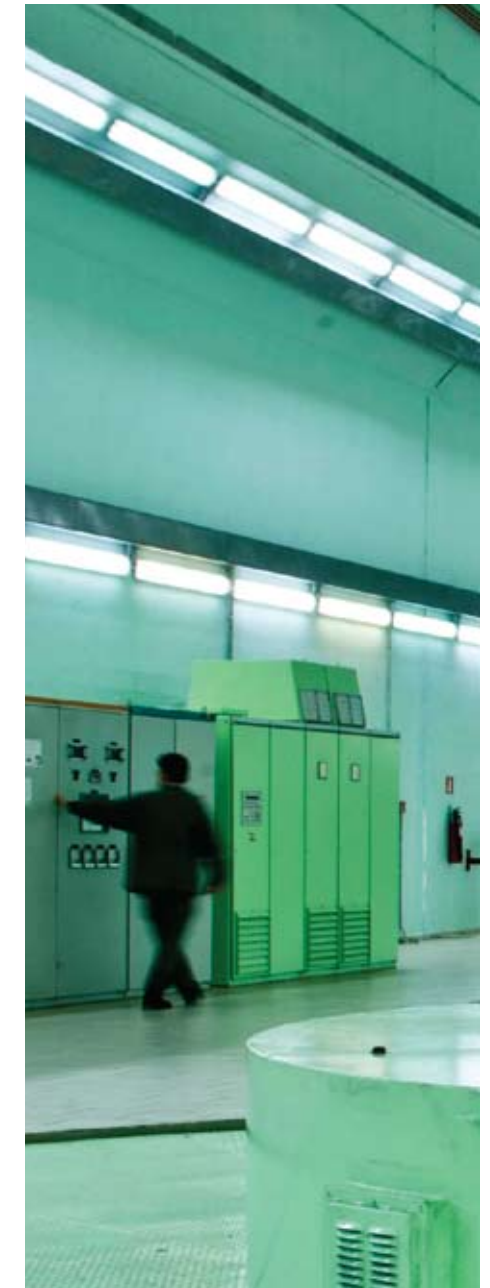
Platanovrysi HPP, Nestos River
