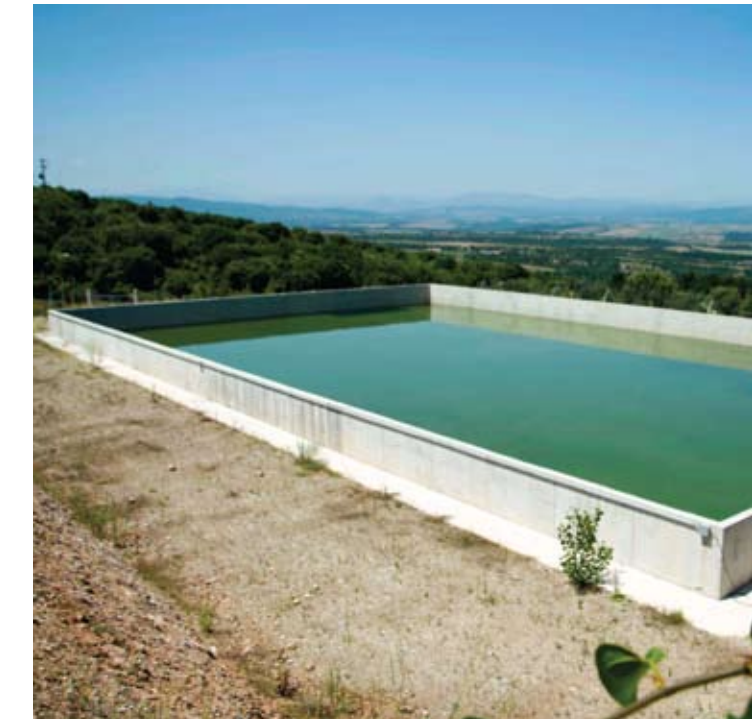
New water supply tank in the Local Community of Paliouria of the Municipality of Deskati
